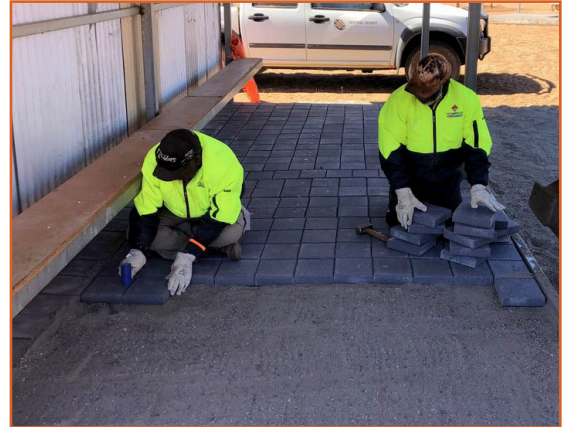
The Engawala Works team paving one of three shade structures for the softball field.
