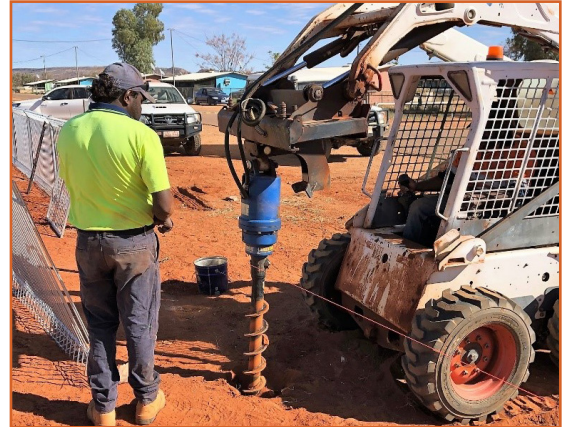
CDRC works crew and the Community Development Program digging post holes for the new park fence.
